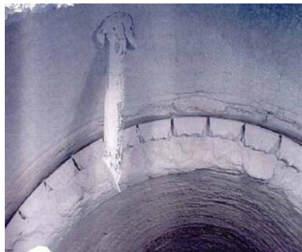
Limestone Injection Pipe
