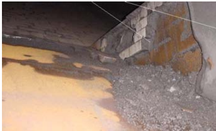
Failed Tile Areas
