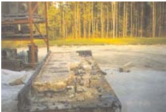
FURNACE DOOR "BEFORE"
