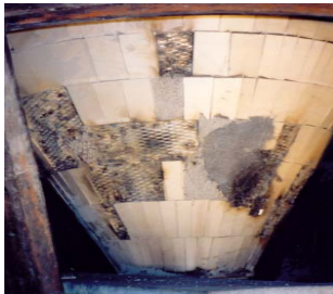
Ongoing tile loss - now repaired with Ceramite® as ongoing system
