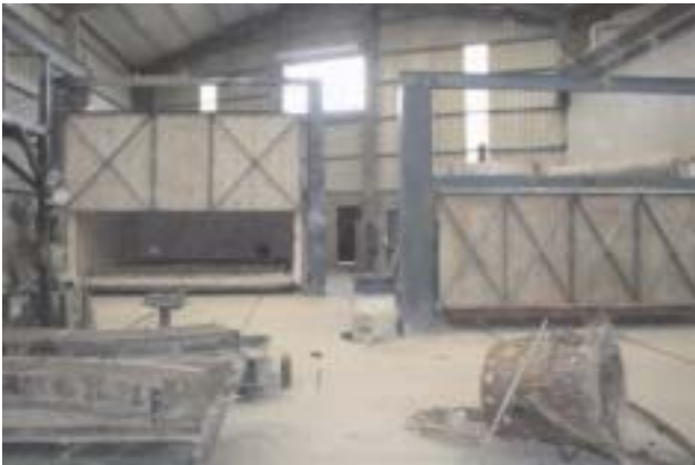
2 Large Drying Ovens
