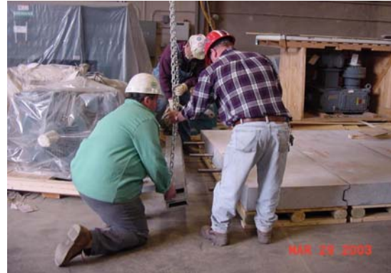
Fabricated Lifting Section Assembly
